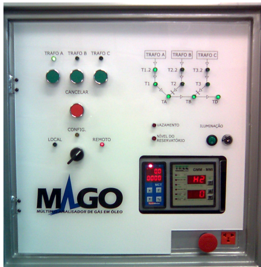
Figura 5. Painel de interface local do MAGO II.
